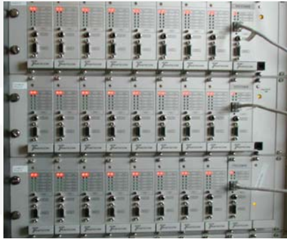
8 VIP boards integrated into a standard 19" rack
