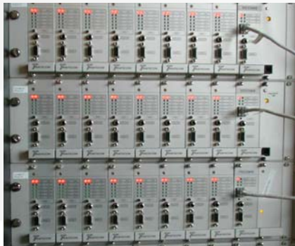
8 VIP boards integrated into a standard 19" rack
